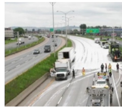
Truck dumps white all over highway in Montreal
